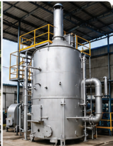
Organic Waste Burnout Equipment
